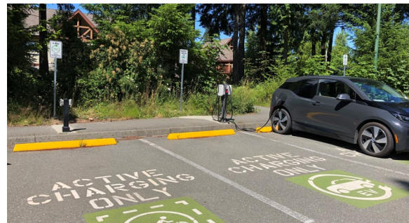
Above: multiple charging stations for electric vehicles have been installed at the campuses.
